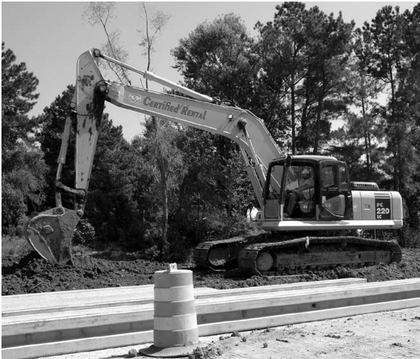
Heavy highway construction is a specialty of Hill Bros. Here, an operator uses one of the company's many PC220LC-7 excavators as part of the Interstate 55 project near Memphis.
