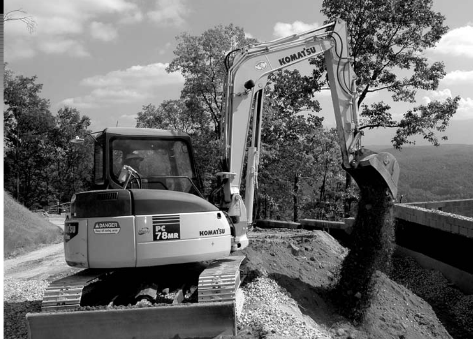
A Gerald Bales and Sons employee uses a Komatsu PC78MR-6 excavator to backfill a foundation on Legacy Mountain. Gerald Bales and Sons has done the entire site preparation for the new housing development and expects to work on the site for many years to come.
