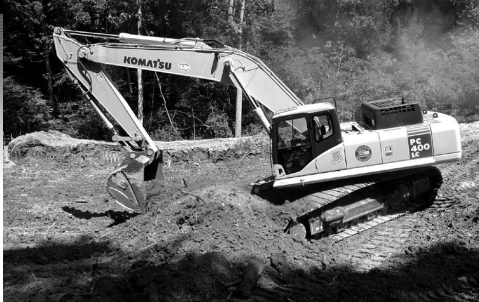
A Farris Excavating operator works a Komatsu PC400LC excavator at a jobsite. "I don't know all the excavators out there, but I've run quite a few of them," said Owner Tyler Farris. "I prefer Komatsu."
