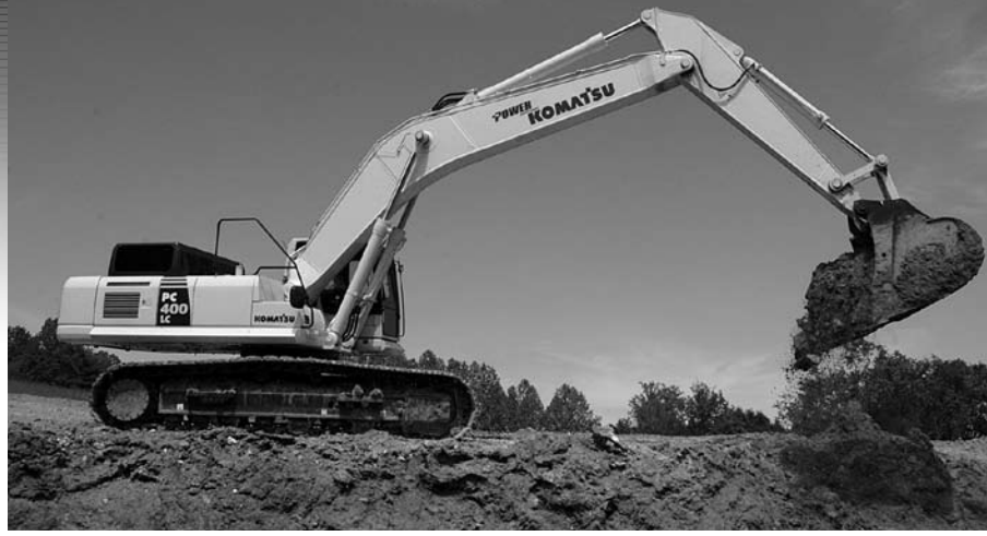
Claiborne Hauling Contractors acquired its Komatsu PC400LC excavators after experiencing success with its PC300s. "We went in and bought a PC400 to see what it would do and it struck the bell on every note," said Grading Division Manager Chris Etters.
