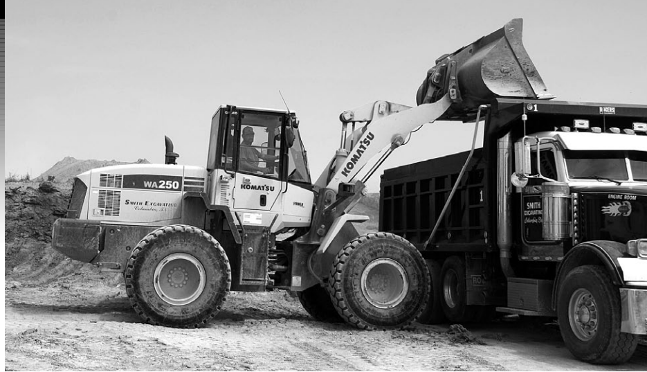
Smith Excavating uses Komatsu machinery, including this WA250 wheel loader for backfilling, carrying materials and pipe, and lifting tracks.
