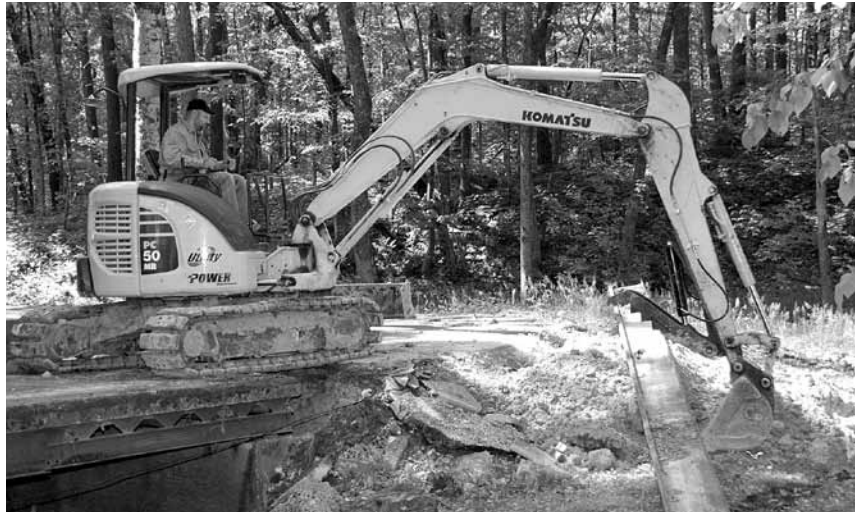
For tight areas where a larger excavator won't work, such as a bridge over a small stream crossing, Bobby Swanson Construction uses this PC50MR-3. "It provides good digging power. It's a very versatile machine because we can also use it in open areas for a variety of tasks, such as dressing up a building pad or digging footings," said Owner Chad Swanson.
