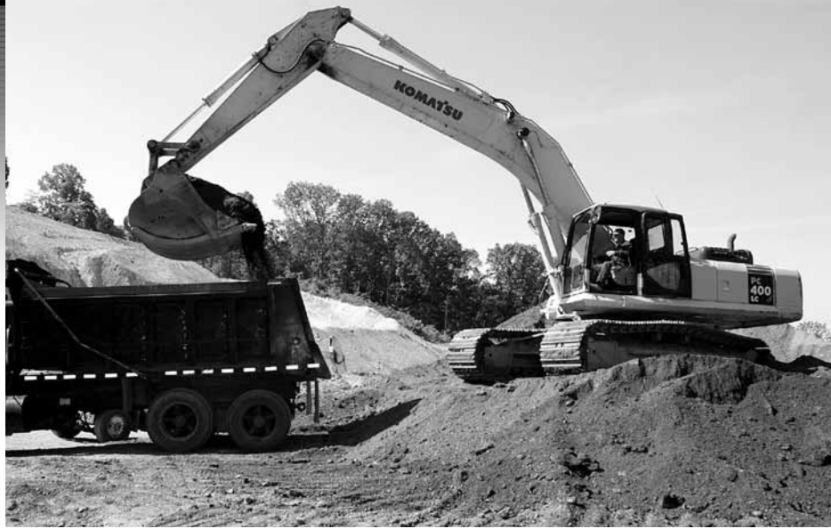
Bobby Swanson Construction recently opened a material pit near its home base of Graysville, Ga., where the company uses its Komatsu PC400LC-7 excavator to load its own trucks along with other contractors' trucks.
