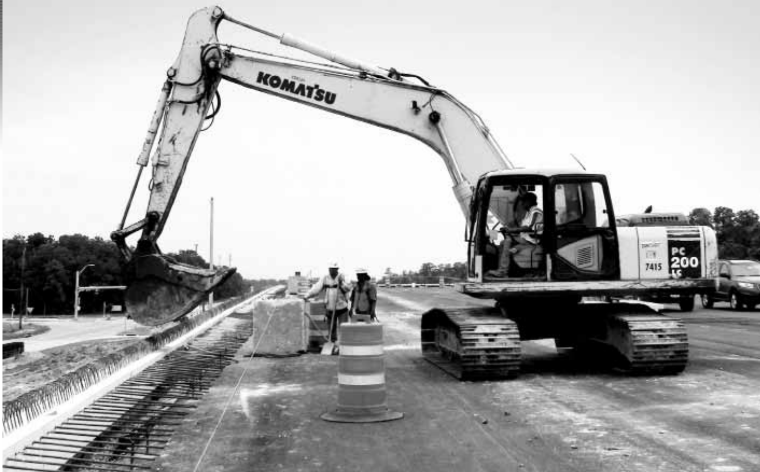
The nation's Federal Highway Program turned 100 last year, and the U.S. continues to work to rehab, rebuild and construct new roads. Today's annual spending on such projects is near what the entire Interstate system cost to build.
