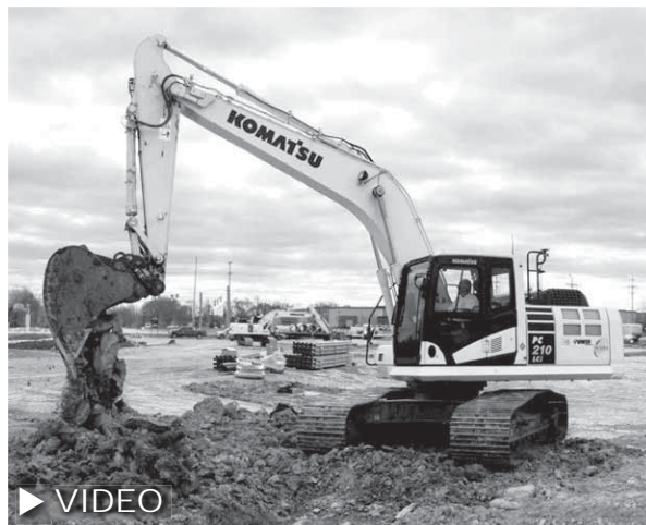
This Grade A Construction operator digs a utility trench with a Komatsu intelligent Machine Control PC210LCi-10 excavator on a 17-acre commercial site in Murfreesboro. “It eliminates overexcavation, so there is no costly material replacement,” said Vice President of Operations Lance Lannom. “We also don’t need someone to constantly check grade, so that person is now freed up to do more productive work.”
