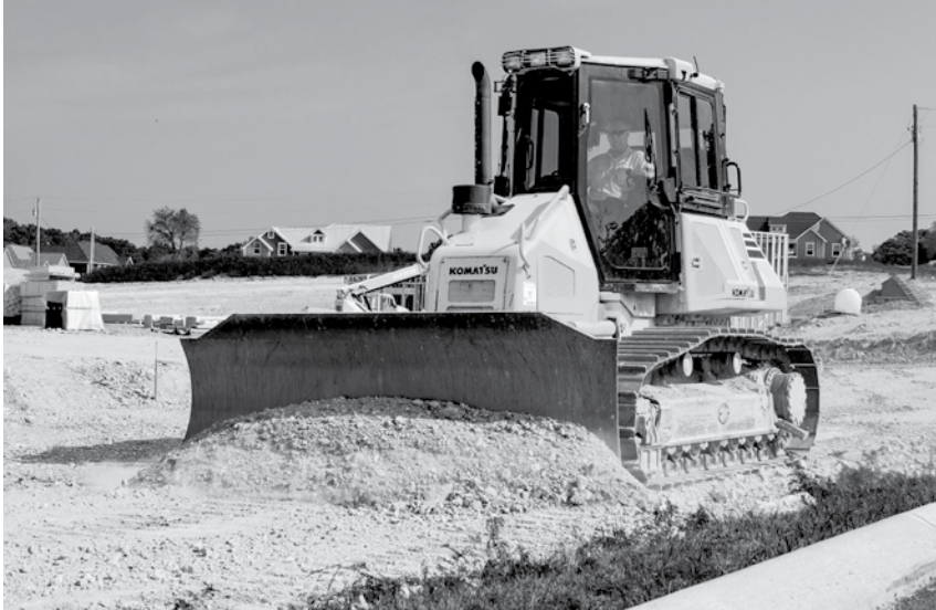
Co-owner Ricky Williams uses a Komatsu D51EX dozer to grade at the company's development in White Bluff, Tenn.
