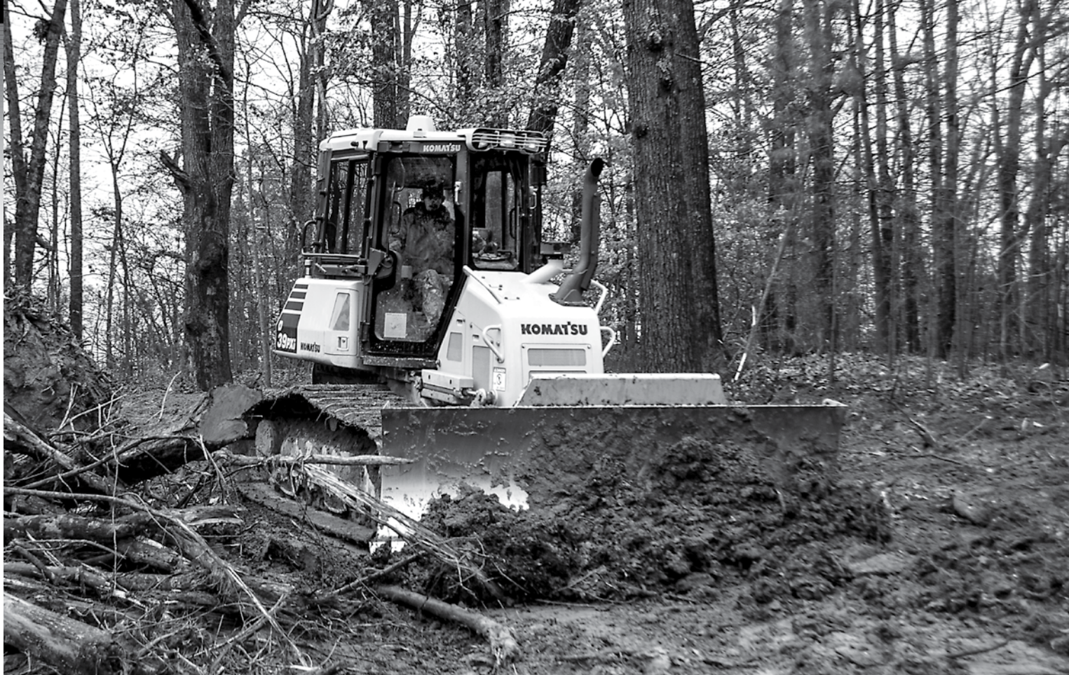
Using a Komatsu intelligent Machine Control D39PXi dozer, a Miller Contractors operator grades a residential lot at the Oakmont Woods subdivision in Jackson, Tenn. “(The D39PXi) expands our operator pool,” said Co-owner Collin Miller. “We have more people now who can jump in the cab and grade a site.”
