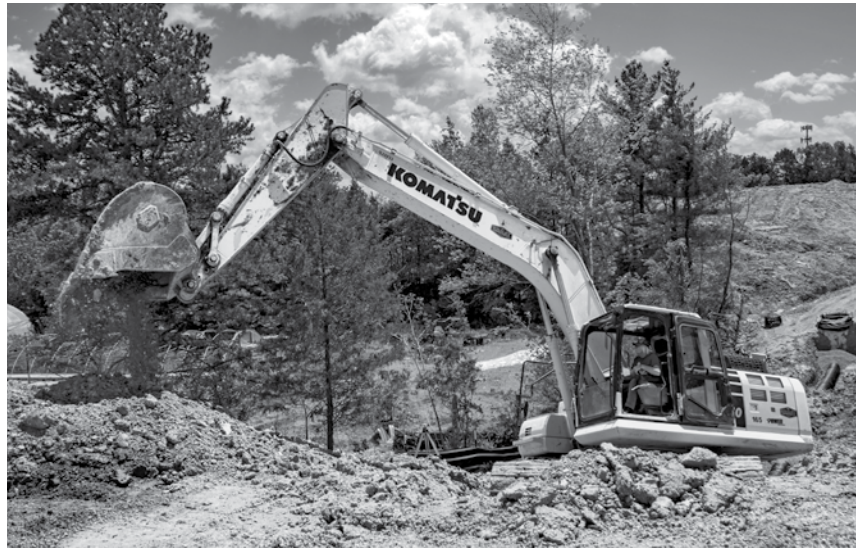
Komatsu excavators, like this PC240LC, are a favorite among Whaley Construction operators for their dependability, handling and cycle speeds, according to President Matt Whaley.
