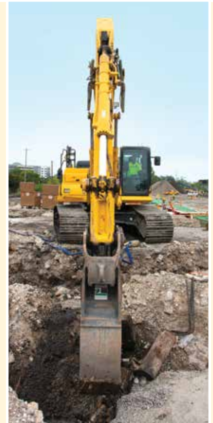
A CornerStone One, LLC operator digs with a Komatsu intelligent Machine Control (iMC) PC360LCi-11 excavator at Komatsu's future global mining headquarters. "With iMC, you can put them right to grade, and once you reach target elevation, it prevents you from overexcavating," said CornerStone One Earthwork Division Manager Scott Christman.
