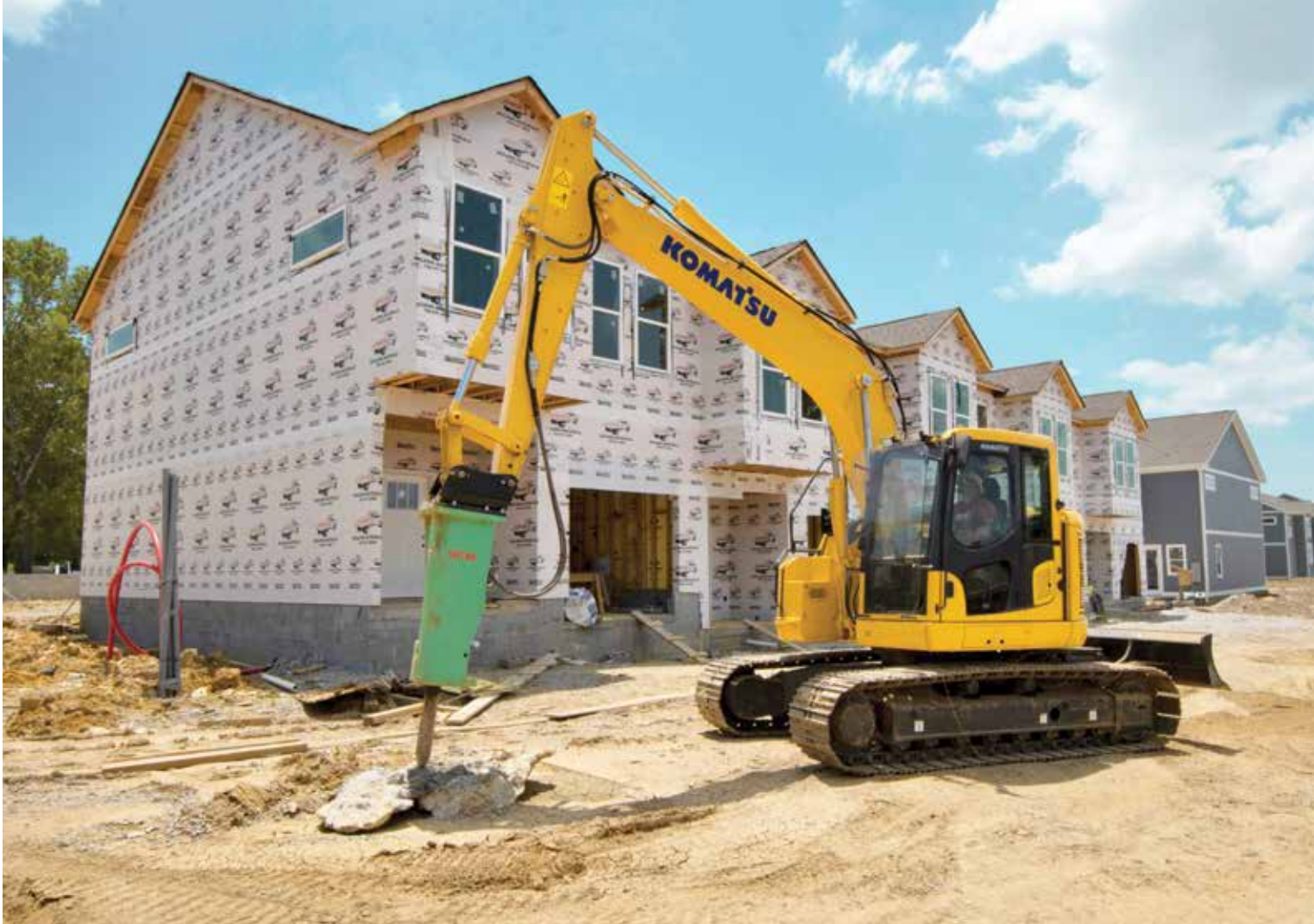
An operator breaks up concrete with a Komatsu PC138USLC excavator that has a Montabert 501 NG hydraulic rock breaker attachment.
