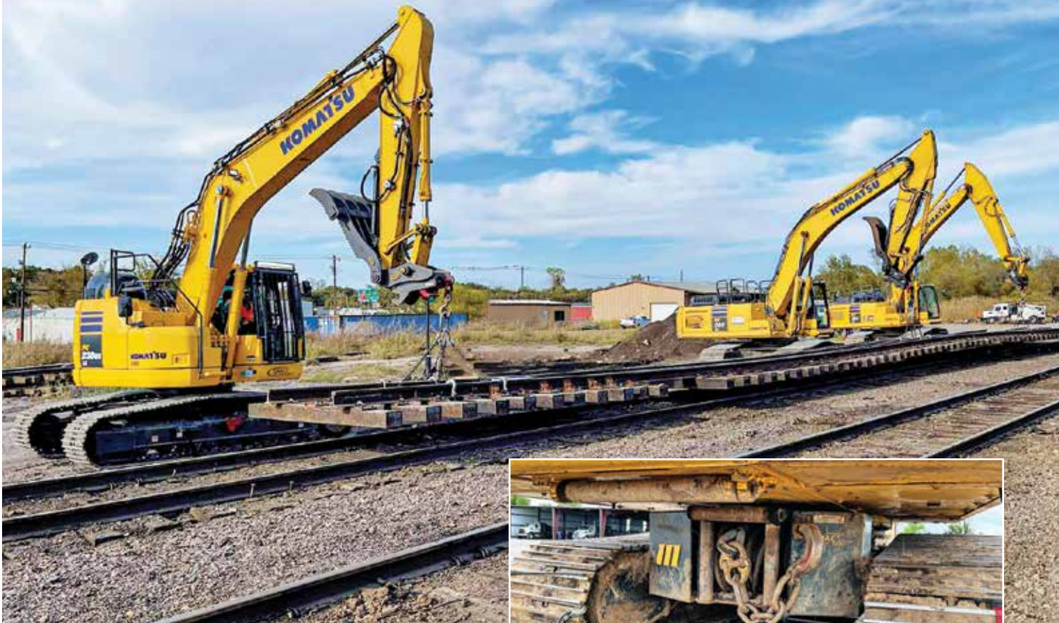
Operators use a Komatsu PC238USLC-11 excavator and two Komatsu PC360LC-11 excavators to lay railway tracks. While one of the PC360LC-11 excavators is standard, the other is upfitted with a recovery winch mounted to the track frame for train wrecks.
