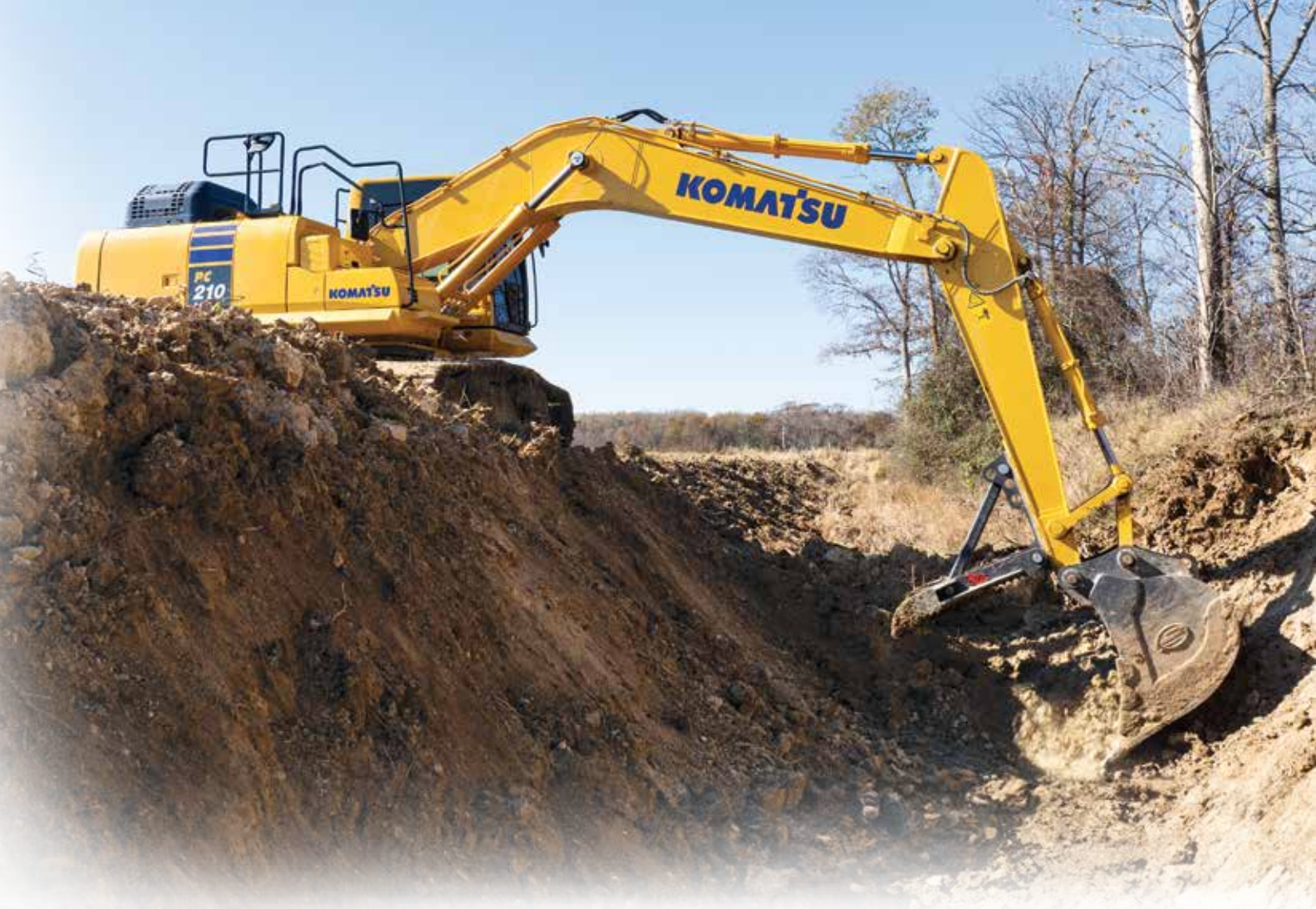
An operator cuts material out of a ditch to widen a levy at a local Arkansas farm with a Komatsu PC210LC-11 excavator.
