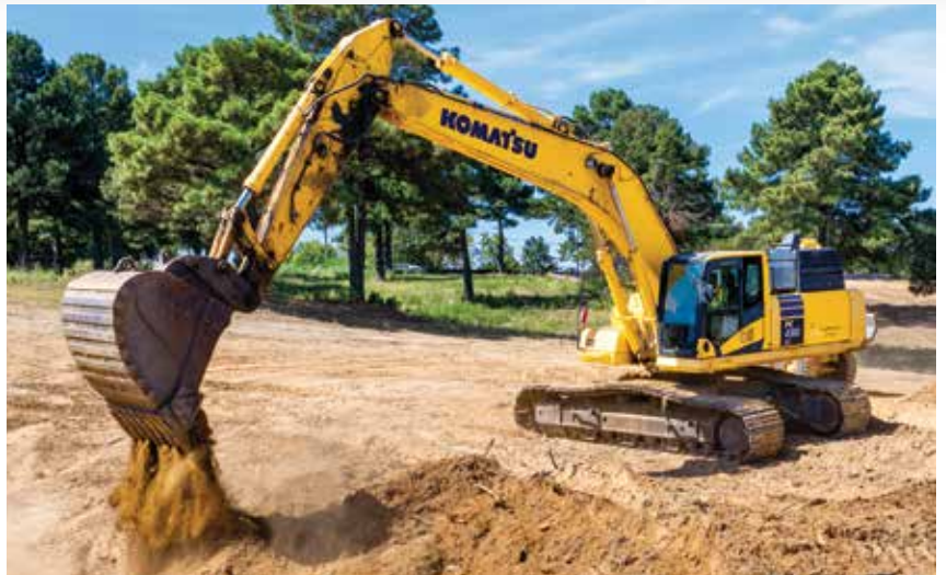
An operator places material into a pile with a Komatsu PC490LC-11 excavator.
