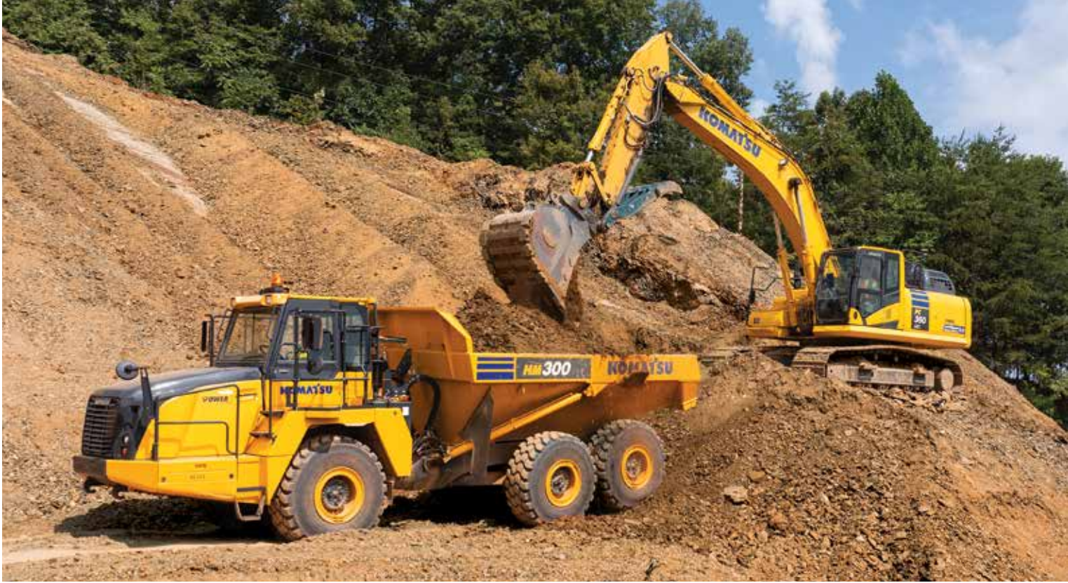
To build an access road, an operator uses a Komatsu PC360LCi-11 IMC excavator to load material into a Komatsu HM300 articulated truck.
